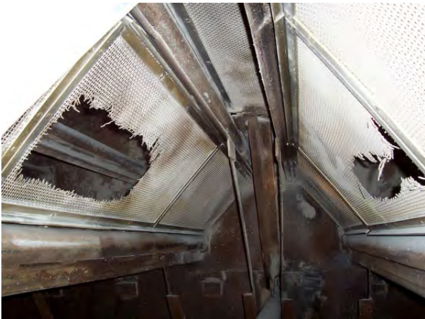
Damaged LPA Screen Material
